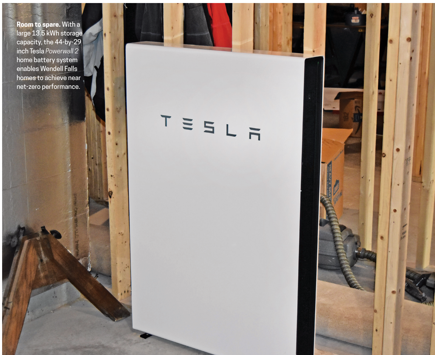
COURTESY OF SOUTHERN ENERGY MANAGEMENT
